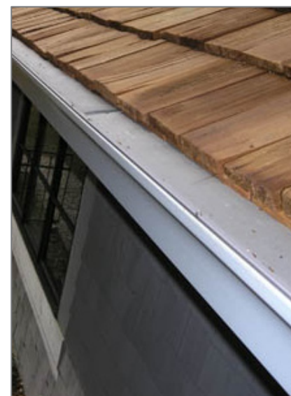
This gutter is covered by a fine mesh gutter guard to keep debris out. Courtesy of Gutter Glove
